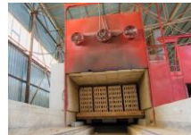
Heat Treatment Furnace
